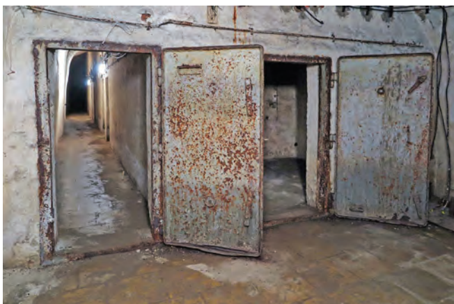
The entrance to the protected control rooms of the wartime aircraft factory
